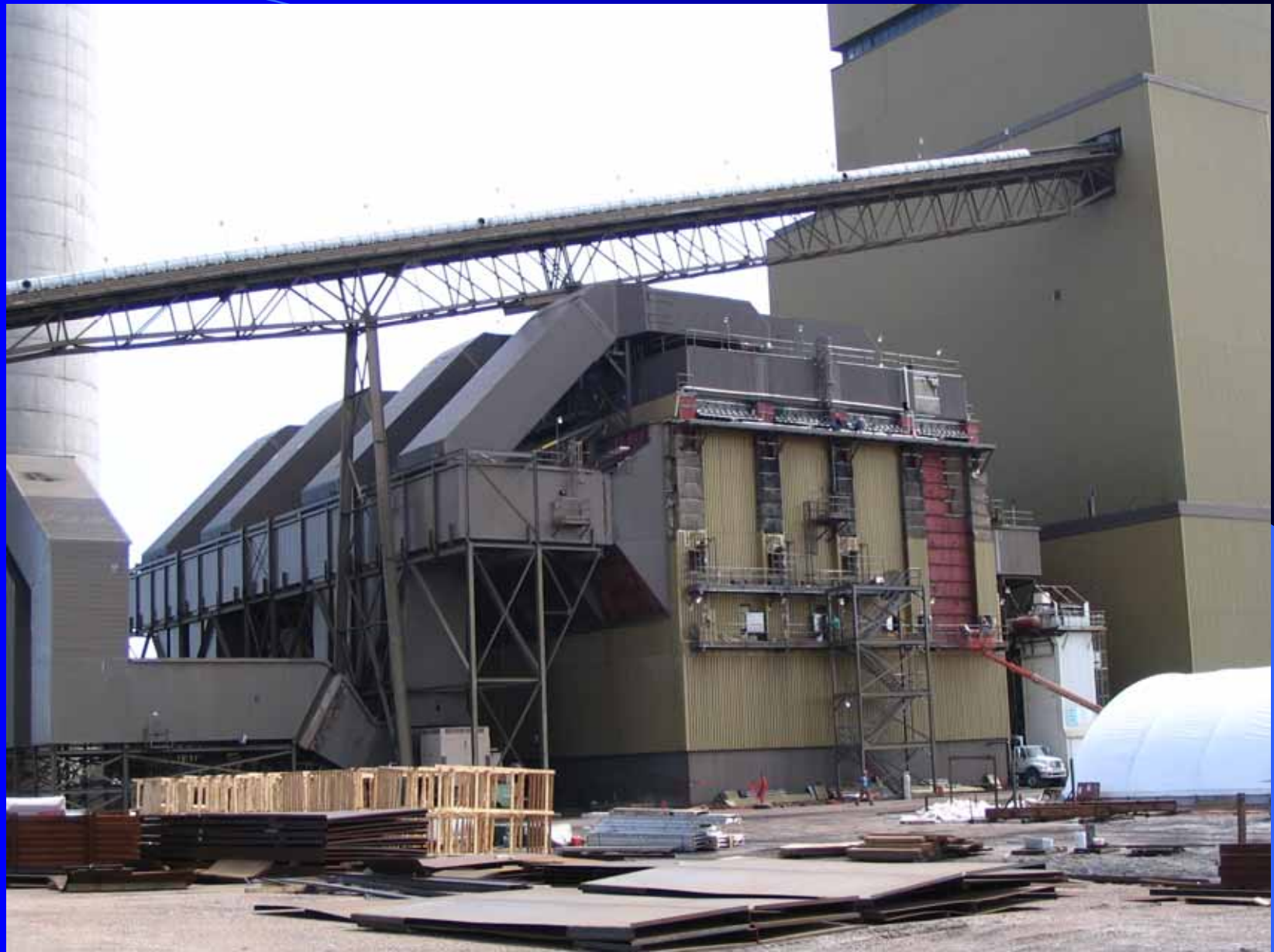
Big Stone Unit 1, Four Parallel ESP Chambers
