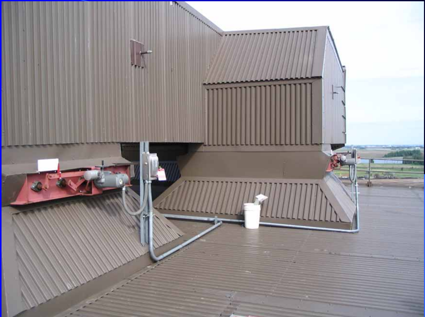
Outlet Plenum Vaned Dampers
