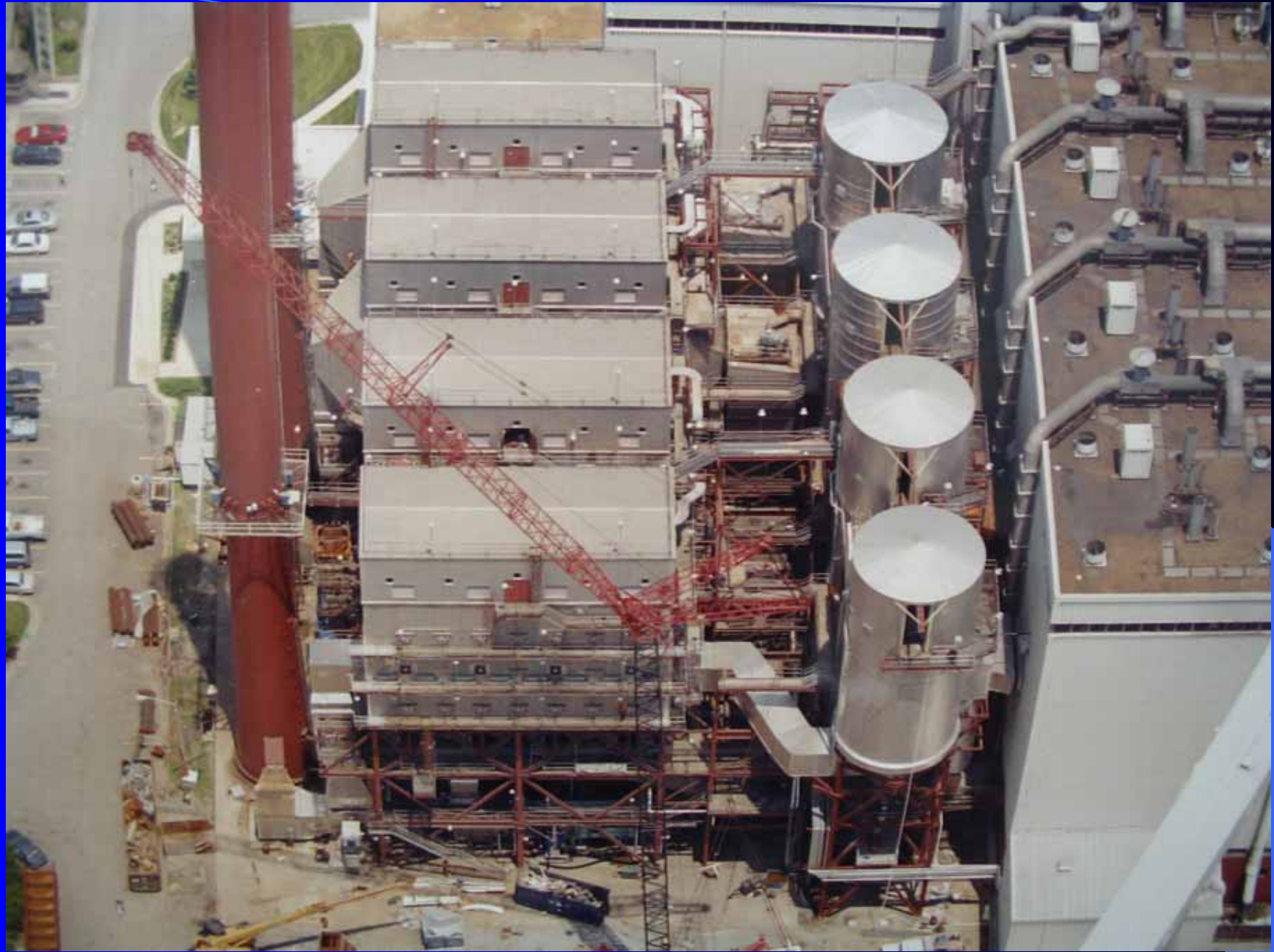
Southeastern Public Service Authority, VA, ESP to FF Conversion
